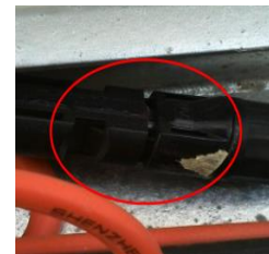
The cable is loose
